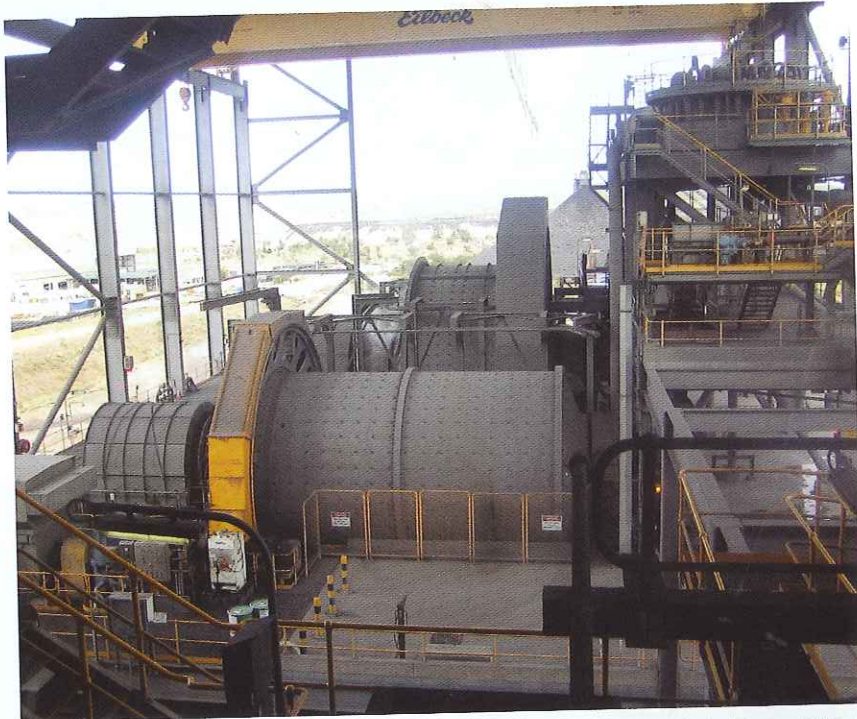
Optimal performance of a SAG mill can be achieved by using an existing Distributed Control System (DCS) or Programmable Logic Controller (PLCs). There should be no need to turn to third-party solutions.
